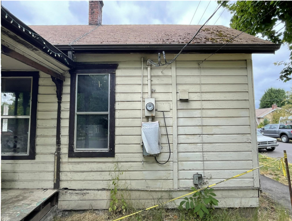
FRONT OF HOUSE SHOWING JOINT AT PREVIOUS ADDITION TO HOUSE
