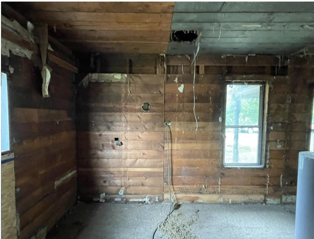
INTERIOR OF LIVING ROOM SHOWING LINE IN FINISHES AT PREVIOUS ADDITION TO HOUSE
