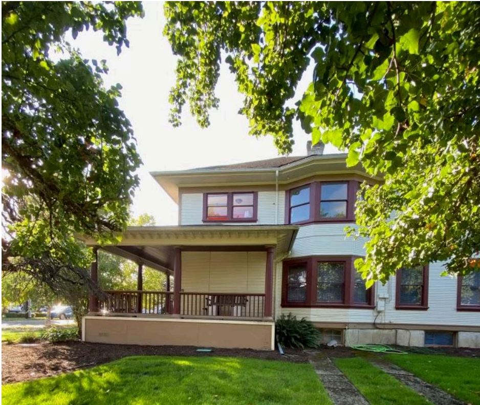
PHOTO 4: Plywood placed over porch piers and no visible skirting, 2024
