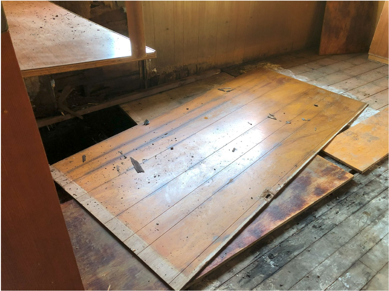
Damage from water intrusion dining area
