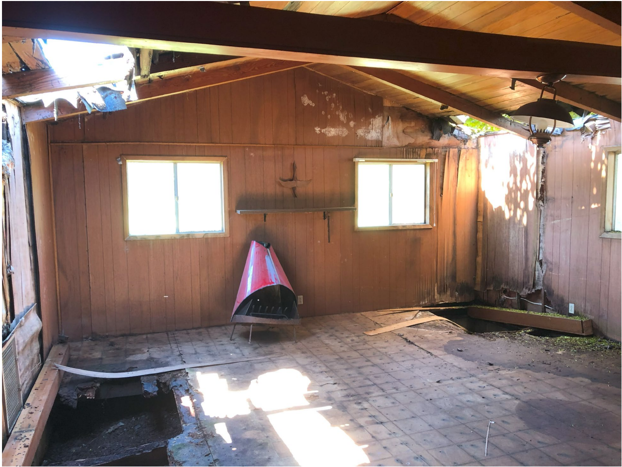
Damage from water intrusion, family room addition
