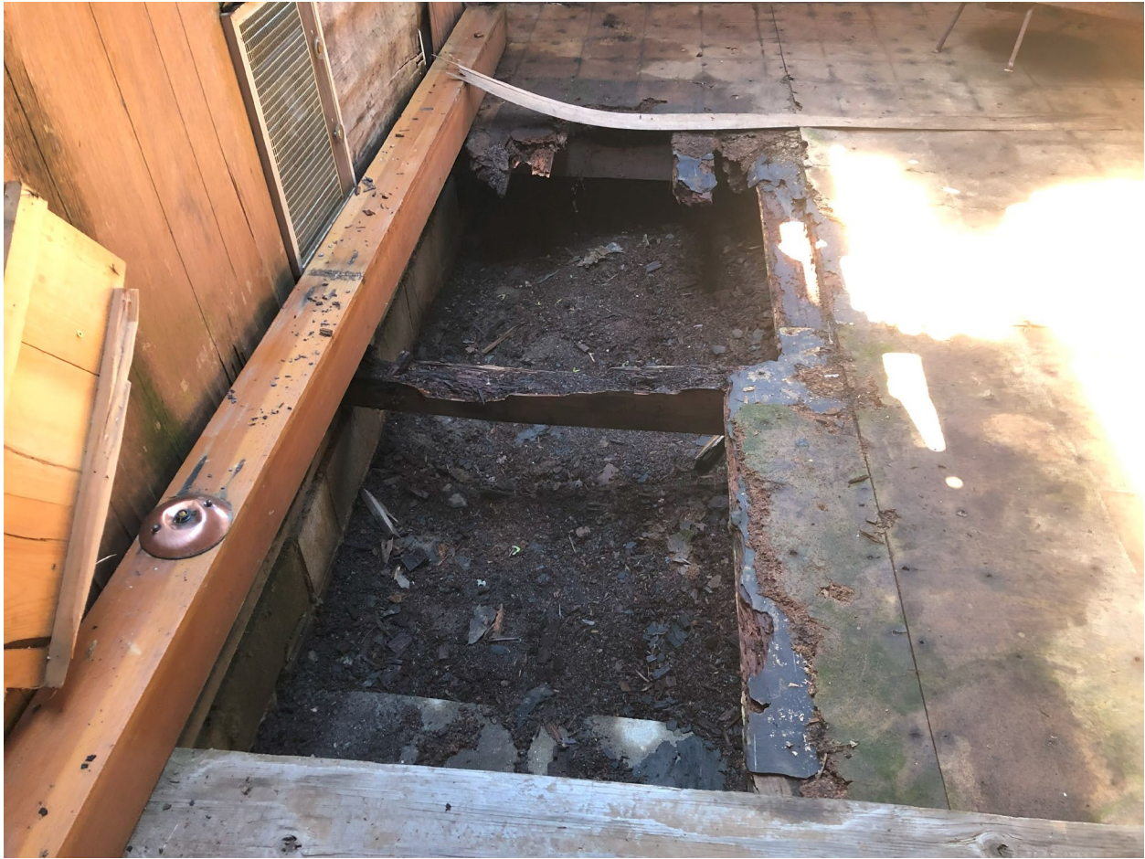
Damage from water intrusion family room addition
