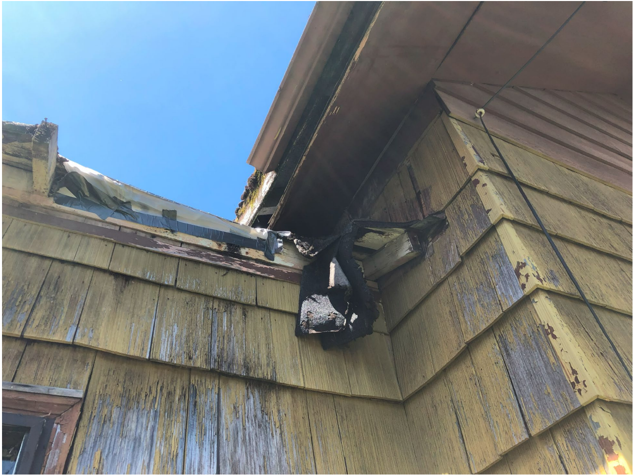
Damage from water intrusion corner of porch addition
