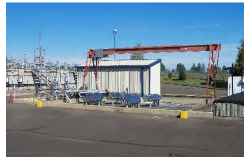
An updated and expanded ultraviolet (UV) system, which uses ultraviolet light to disinfect the treated water and returns it to the receiving stream (South Yamhill River).
