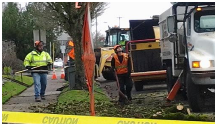
Jeff Hendricks, left, Parks Maintenance (11 years), removing hazardous tree at the Chamber of Commerce.
