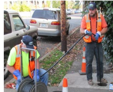
City Conveyance System crew performing maintenance on a sewer line on NE 4th Street. – pictured Utility Worker II Randy Clow & Sr Utility Worker Matt Bernards
