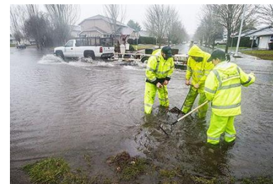
Kristine Reed, right, Parks Maintenance (13 years), clearing storm drain during December 2015 rains.
