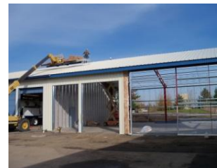
Haworth Inc. constructs the Conveyance Building addition which will house the new Vac-con and excavation equipment.
