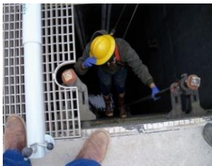
Mechanic, Dave Allen, repairs basin de-watering valves. This vault is 36 ft. deep and contains 6 valves which drain plant process tanks.
