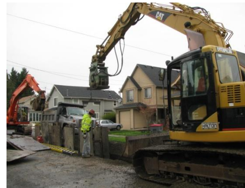
Work on the Downtown Basin I&I reduction project began in March of 2012.
