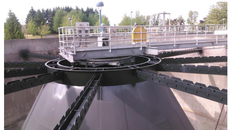
The City continued to invest in upgrades to the public sanitary sewer system in 2019. Work included recoating of tertiary clarifiers #1 & #2 and ATAD #3 at the Water Reclamation Facility.
