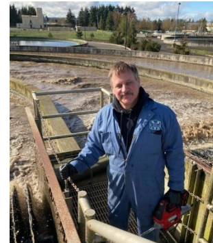
As part of the preventive maintenance program, mechanic David Chitwood, who prefers Joey, is greasing shaft bearings on one of the oxidation ditches.
