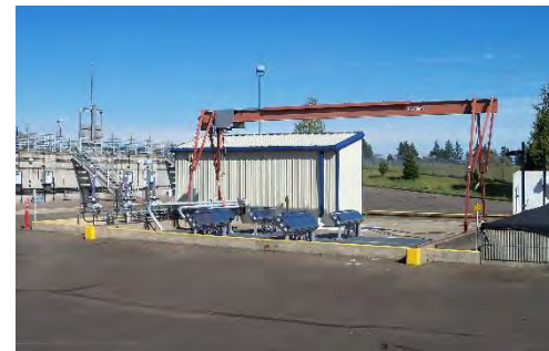
An updated and expanded ultraviolet (UV) system, which uses ultraviolet light to disinfect the treated water and returns it to the receiving stream (South Yamhill River).
