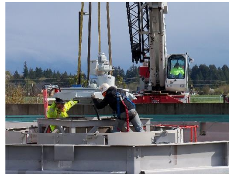
A crew from Stettler Construction uses a crane to install a drive assembly into secondary clarifier #3.
